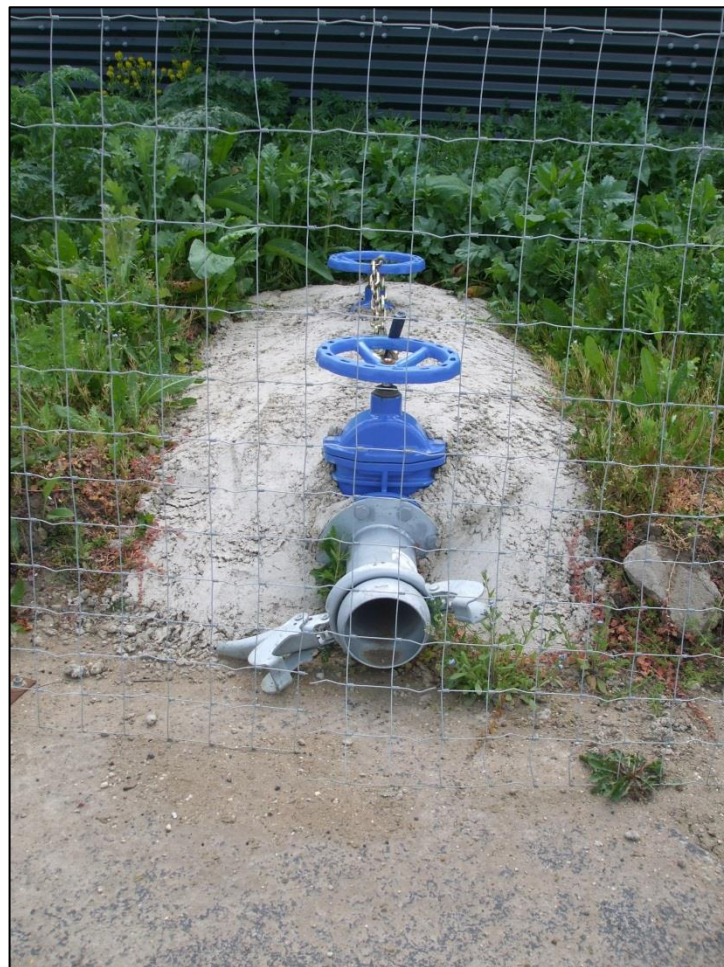
Tanker/Tank discharge point
